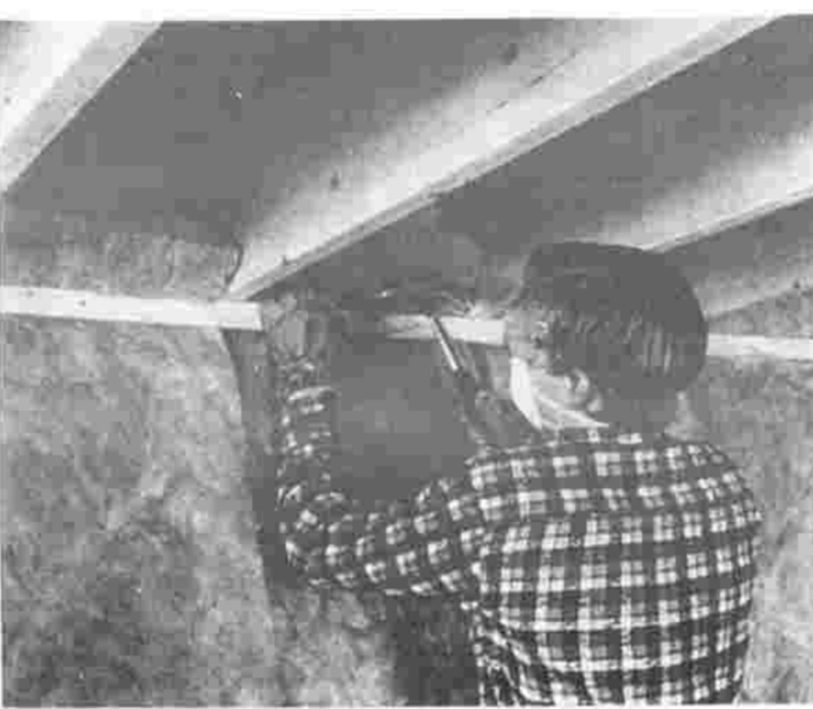
TO INCREASE THE ENERGY EFFICIENCY of your home, insulate crawl spaces. The Department of Energy recommends R-19 or 6 inches of fiber glass insulation for crawl spaces in most areas of the country. This homeowner is nailing unfaced insulation blankets to a sill with long furring strips.
